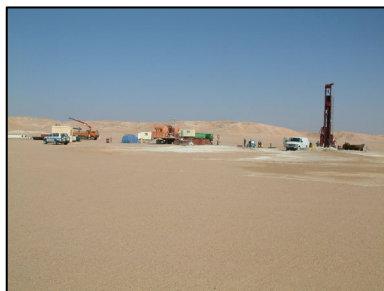
Small mobile, self-contained, drilling units were used to keep the Project on target.
