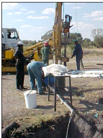
DWA's crawler rig drilling a monitoring borehole to study groundwater levels in the Project Area.
